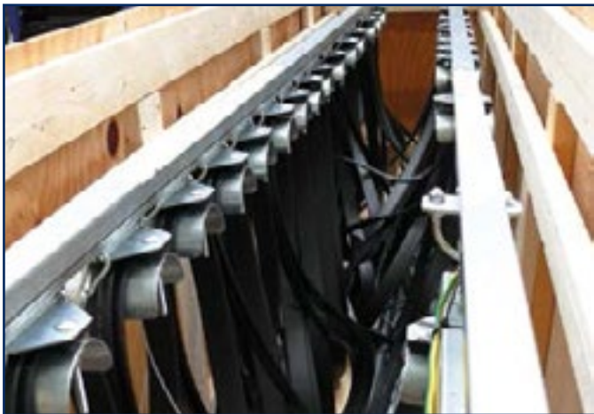
Prewired hoist trolley power supply
