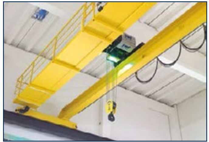
Double girder overhead bridge crane with crane lights
